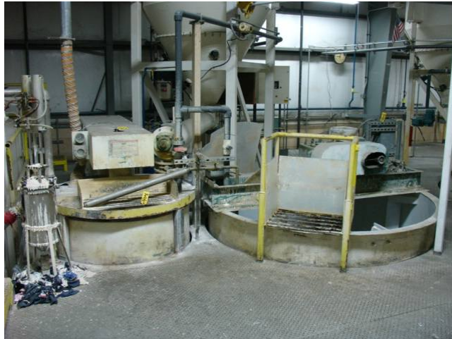
One of two pairs of mixing tanks
